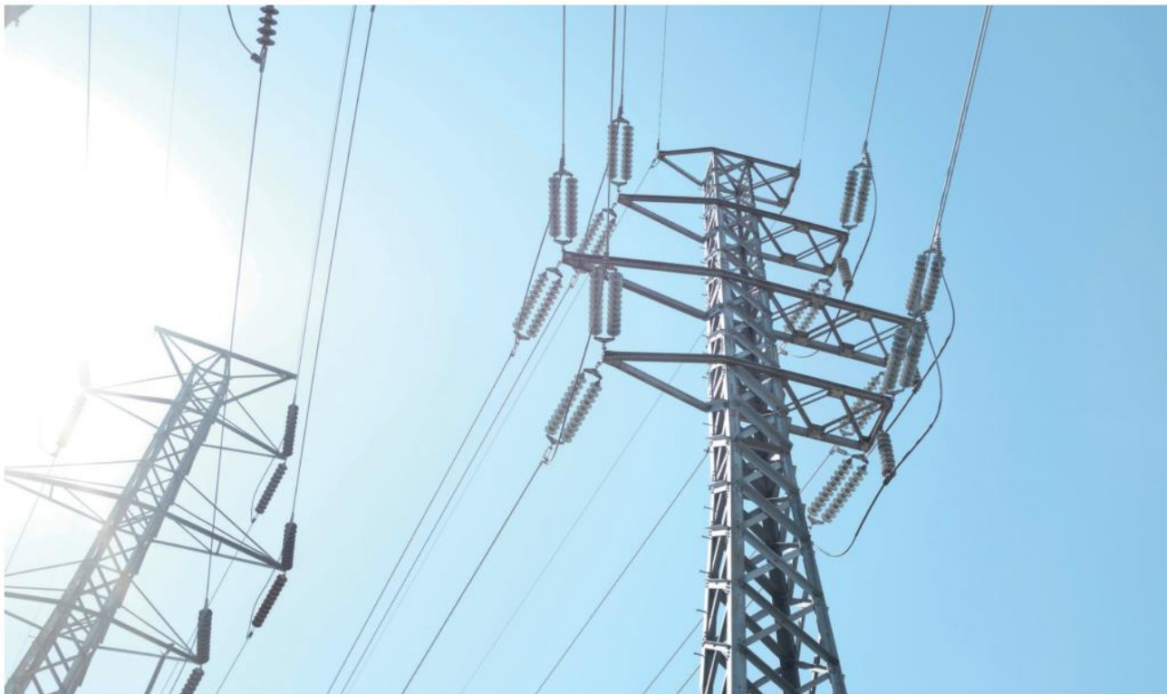
A high-voltage transmission tower: Preparing the grid for RE integration. © Jonathan Hanna via Unsplash
